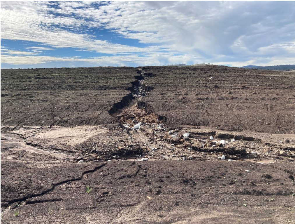
FIGURE 3-1 TOPSOIL EROSION DUE TO RECENT RAINS
